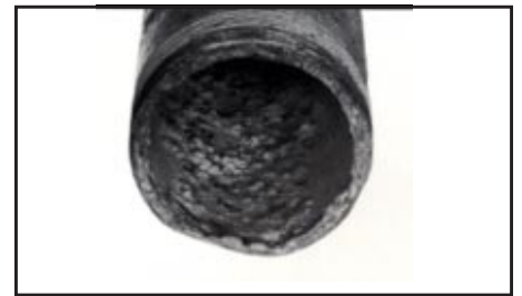
Figure 7-3. Oxygen in the system speeds corrosion (oxidation) of pipes, causing pitting such as shown here.
