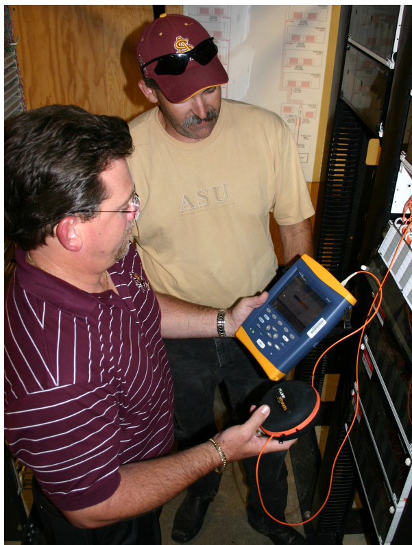
L to R: Craig Trimble, director telecommunication infrastructure IT at ASU, and Tony Janousek of Kearney Electric, one of ASU's contract installers, using the OptiFiber to check the fiber backbone in one of the telecom rooms.
