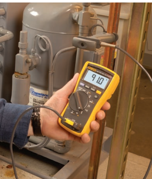
Measuring liquid line temperature with a DMM and a pipe clamp.
