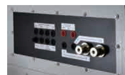
Internal terminals portion
