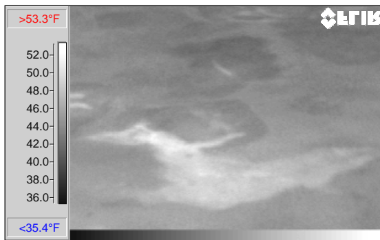
Figure 5. Water saturation pattern on SPF roof
