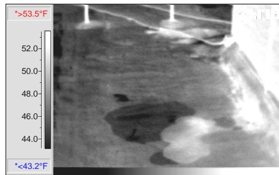
Figure 6. Water saturation pattern on SPF roof
