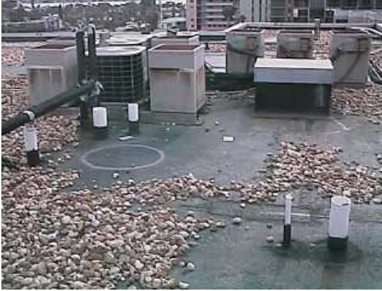
Figure 19. photograph of a partially exposed EPDM membrane
