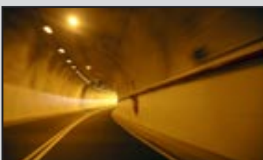
Lighting of tunnels
