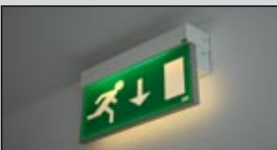
Measuring the emergency lighting in emergency exits
